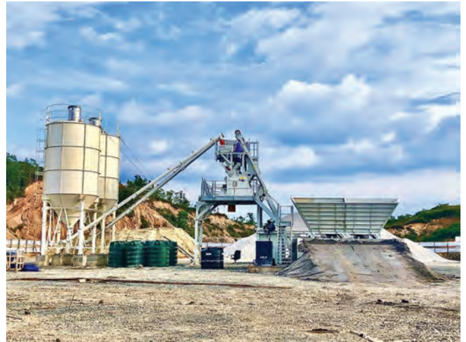
Elba CBT 60 SL concrete plant from Ammann in operation on a housing project in Malaysia.
